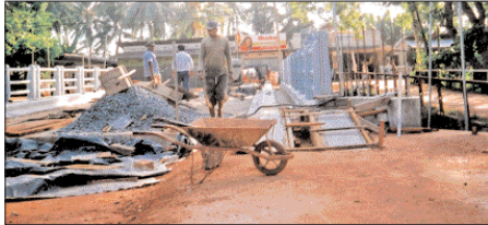
Construction activities of the new Walahapitiya bridge in the Nattandiya electorate costing Rs. 40 million is nearing completion and will be declared open by Highways Minister T.B. Ekanayake shortly. This 60 foot long and 30 foot wide bridge built by the Highways Ministry will solve the transportation problem of nearly 10,000 people in the Muttibandiwiwa, Medagoda, Wetugahamulla and Yatakalawa villages in the electorate. On right is the old dilapidated bridge which is nearly 100 years old. Picture by Antony Fernando, Puttalam District Roving
